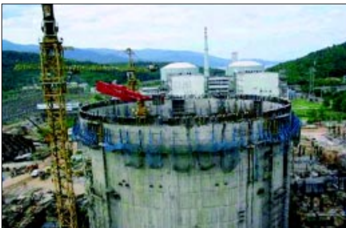
Kaiga Atomic Power Project-3&4
